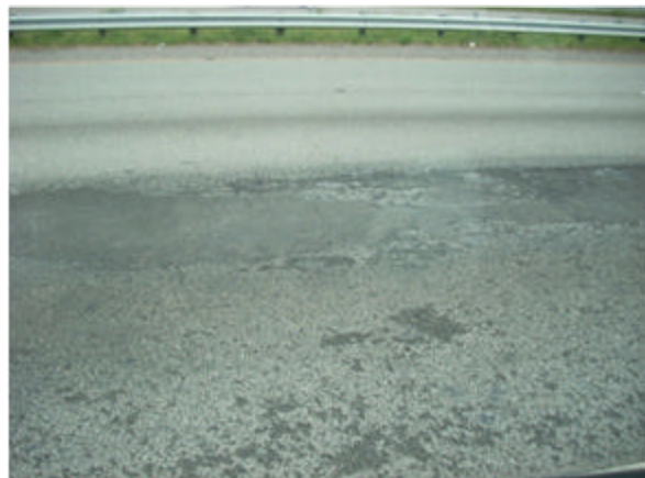
Severe Raveling on OGFC After 42 Months
